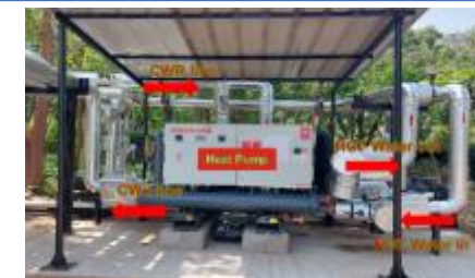
First Plant across Cummins Global Sites to adopt Heat Recovery for Clean Room HVAC systems
